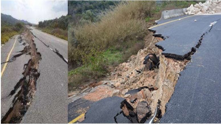
Figure. 3 The Collapse in Al-Haffah diversion
